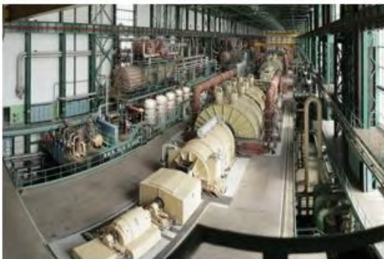
Turbine hall before any dismantling (05/2013)
